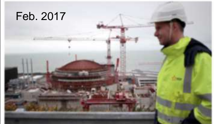
The construction site at Flamanville in northern France. Will it ever be completed? Photo: Charly Triballeau
